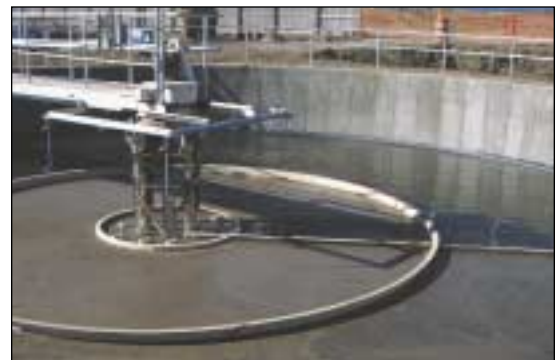
Waste treatment plant. Microbiologists and engineers have successfully harnessed and optimized the use of various microbes to treat sewage and other forms of waste water.
